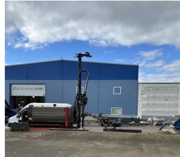
Factory in Markaryd, Sweden: Geothermal heating and renewable fuel
